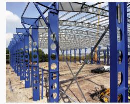
The relatively low self-weight of steel structures reduces material use and deliveries to site
