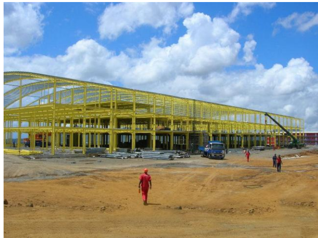
The second sewing factory constructed for CMT by REIDsteel was in Phoenix. It measures 173m x 61m, with three floors. The ground floor is divided into four sections, for washing, printing, cutting and dyeing. The first floor has storage at either end, as well as sections for embroidery and traditional make-up.
